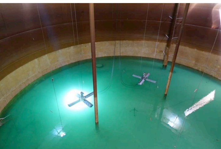
Rosslyne Tank's Two Floating Surface Aerators
