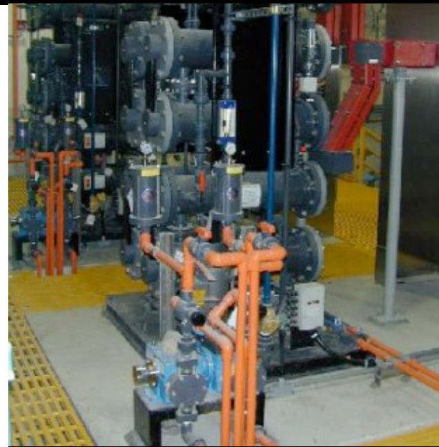
Encore® 700 installations at SNWA
